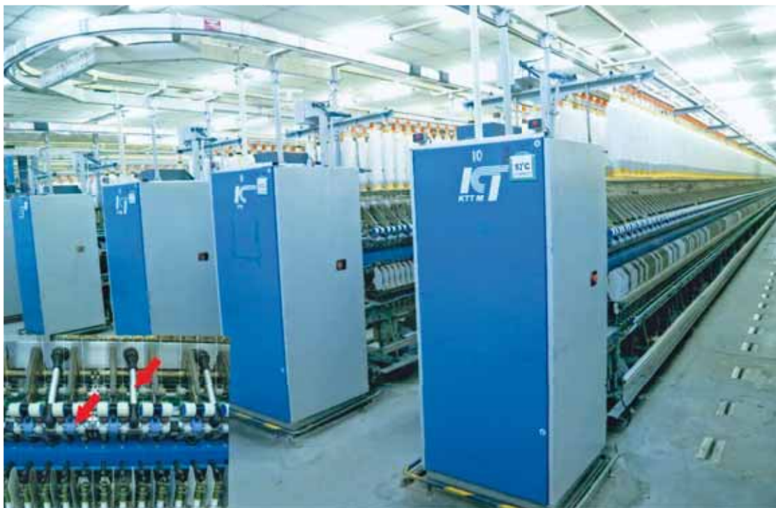
A view of the "Compact System" attached in KTTM Ring Frame during the year in our "A" Mill Spinning Hall at Rajapalaiyam.
