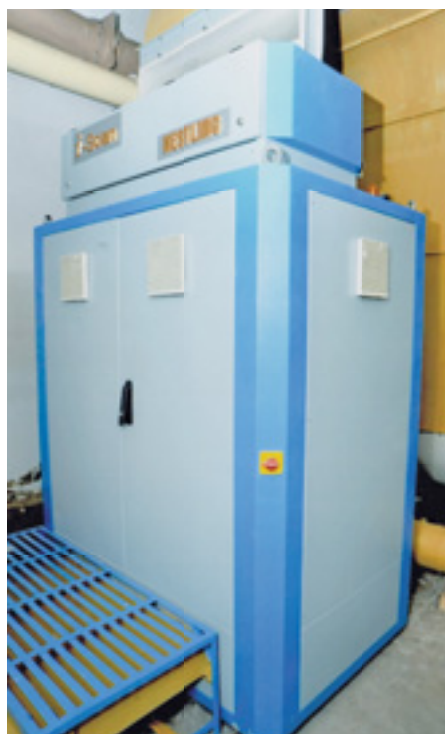
A view of the "I" scan contamination removing machine installed in our "A" Mill Blowroom at Rajapalaiyam.
